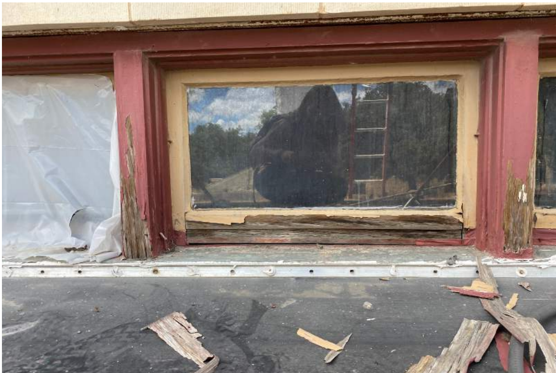
06. Existing Conditions: Woolworth Building ground floor transom window, Houston Street side looking south.
