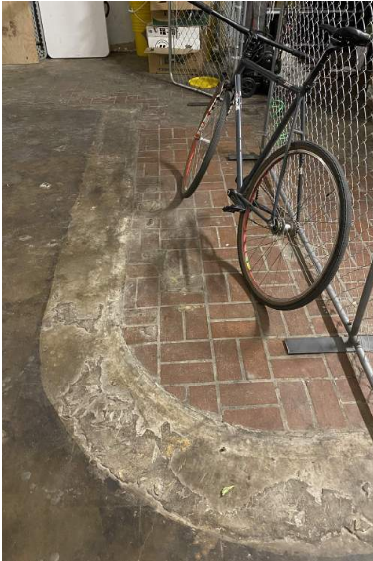
40. Existing Conditions: Woolworth Building Interior first floor, view of lunch counter floor scarring.
