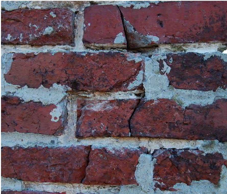
Damage to historic brickwork by Portland cement repointing
