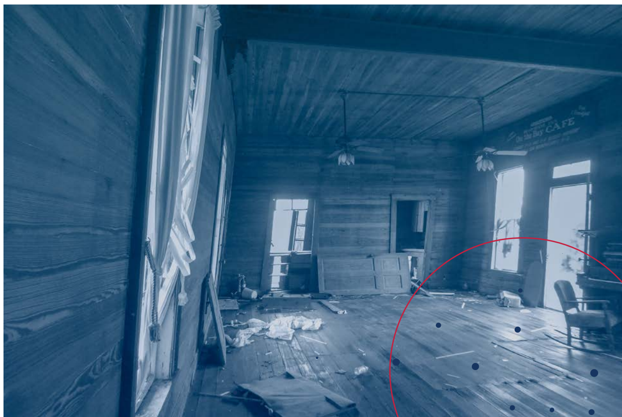
JOHN HOWLAND WOOD HOUSE, BAYSIDE, REFUGIO COUNTY, DAMAGED BY HURRICANE HARVEY
