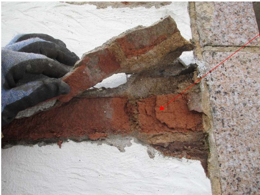
Damaged brick back-up covered by plaster/stucco.
