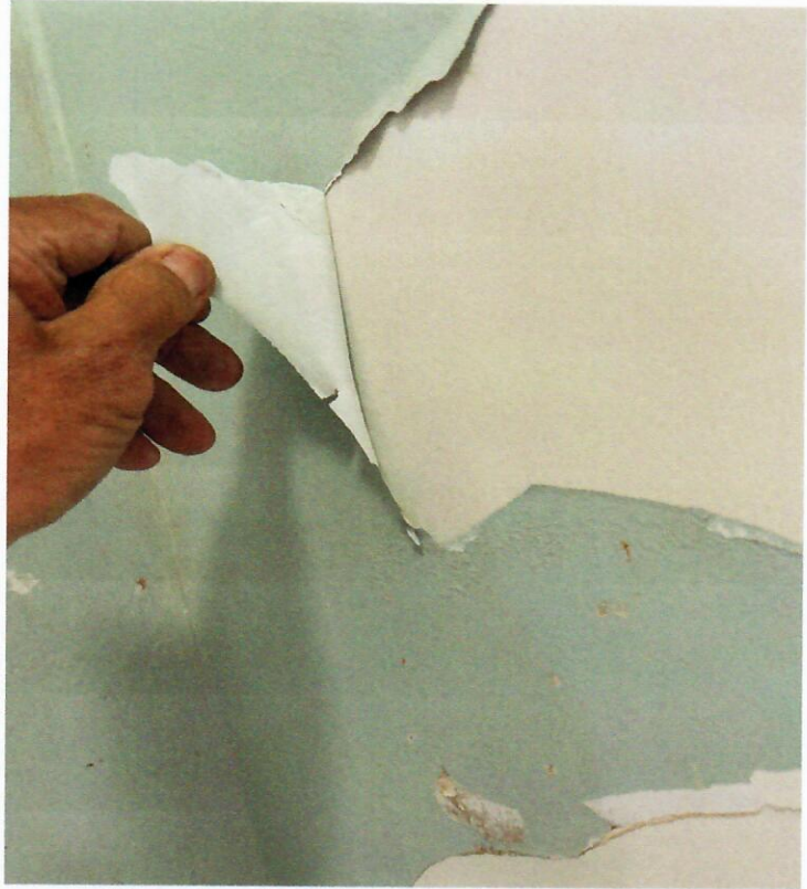
Photo shows lack of paint bonding to drywall muds
